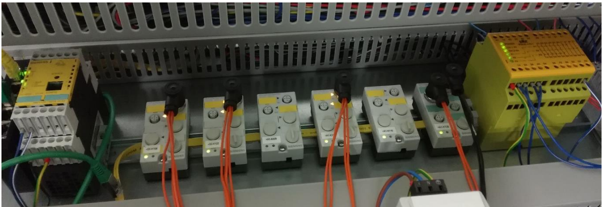
Figure 3-15 Safety Components Mounted in the Electrical Panel
